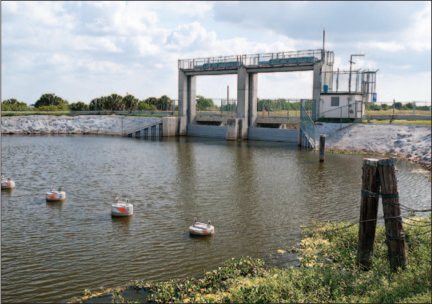
The C-54 structure is one of several water control structures in the Upper St. Johns River Basin that stores and controls storm water.
